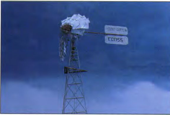
Fig. 2.20 Borehole pump at Khowarib. Courtesy E Marais
