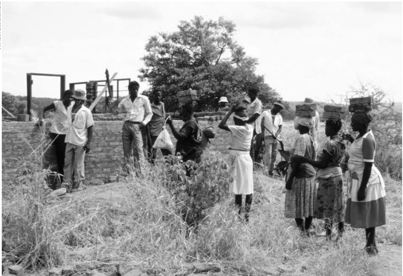
Villagers from Nyenyunga ward construct a teacher's house with their campfire wildlife earnings Gokwe district, Zimbabwe
